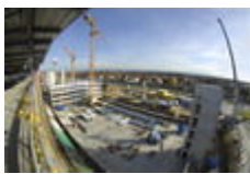
Construction work at the building site to expand the car park at Dresden International Airport
